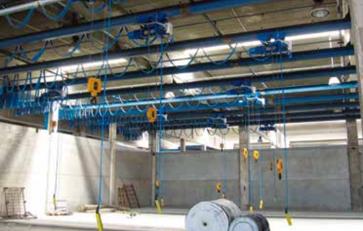
Magazzino trasporto coils - Coils transport warehouse
